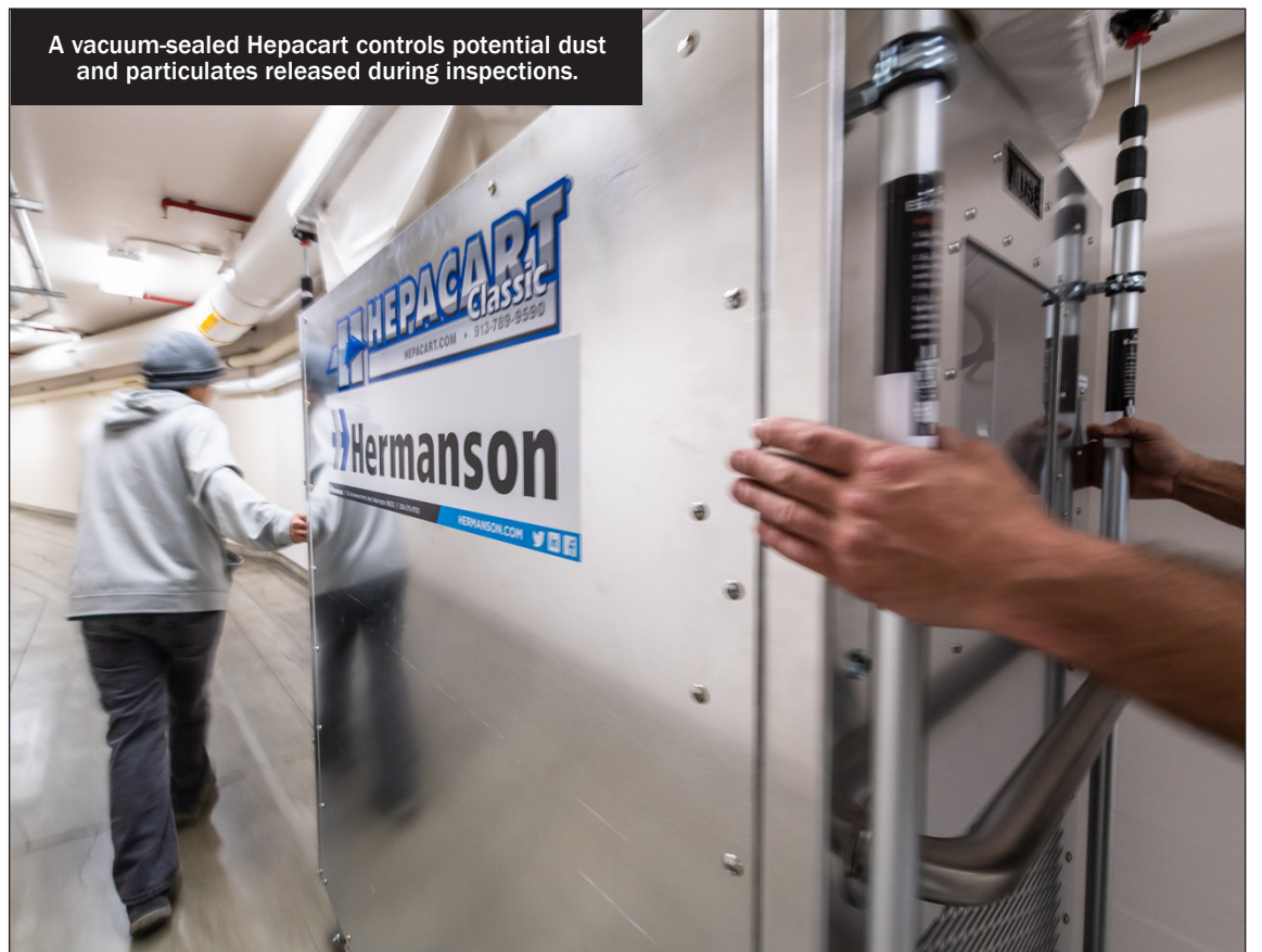
On average 55% of all inspected dampers fail within the first 10 years due to building settling, tenant improvements and other factors.
