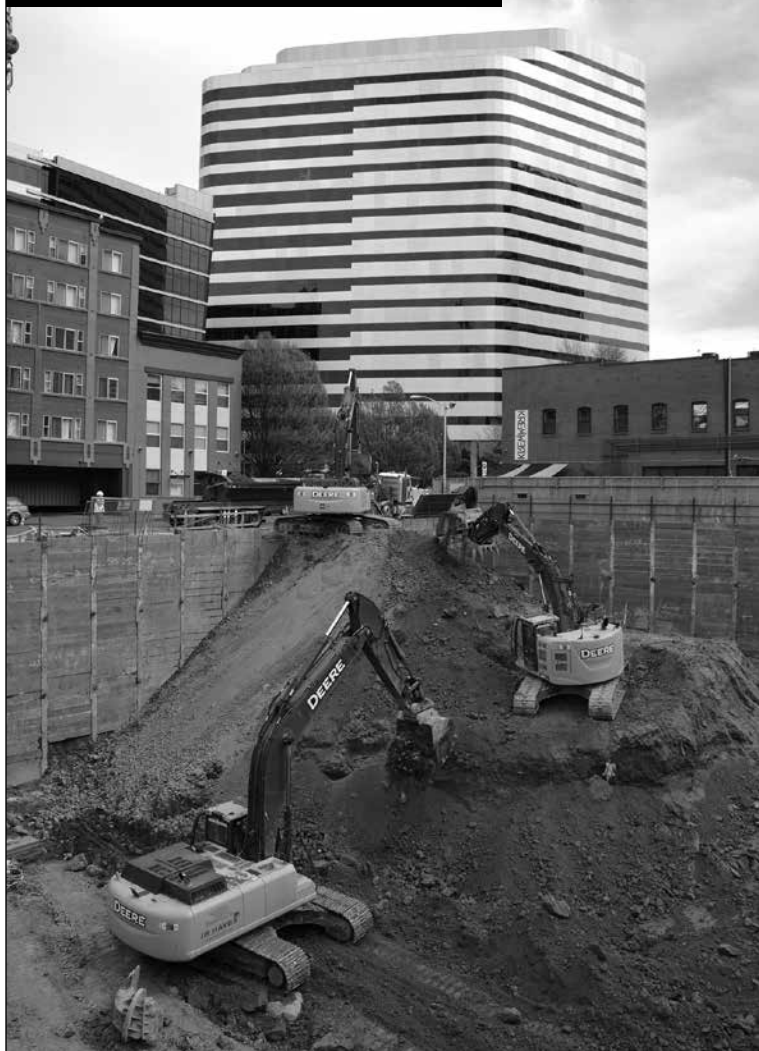
Operators worked together to move dirt out of the Kinects project hole in Seattle.
