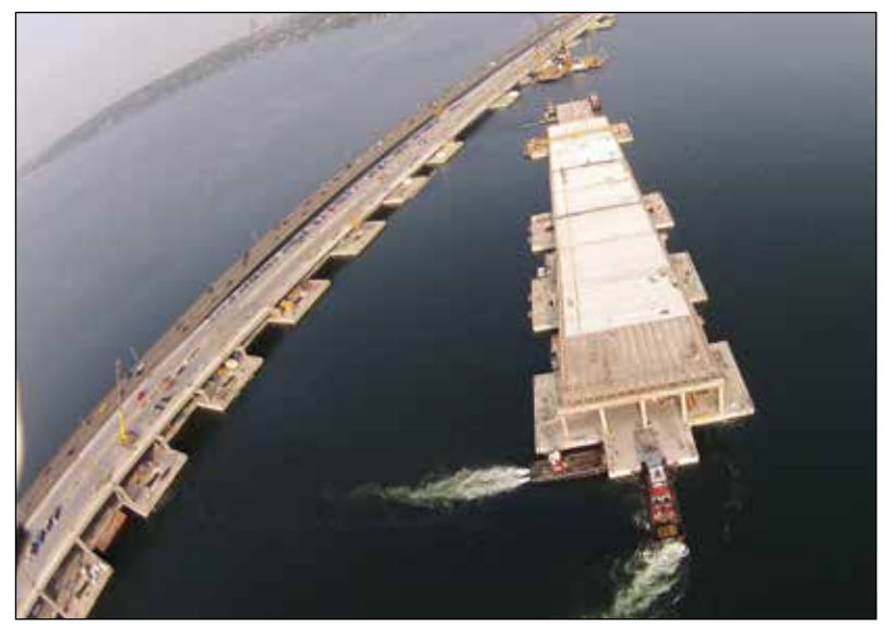
Crews bolted together three pontoons to create a raft, allowing them to work on multiple bridge portions at once.
